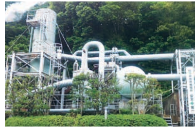
Suginoi Geothermal Power Station
