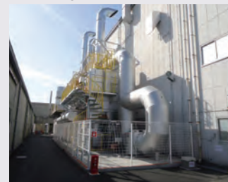
VOC processing equipment (RTO) installed at the Tokyo plant of the Ueda plant
