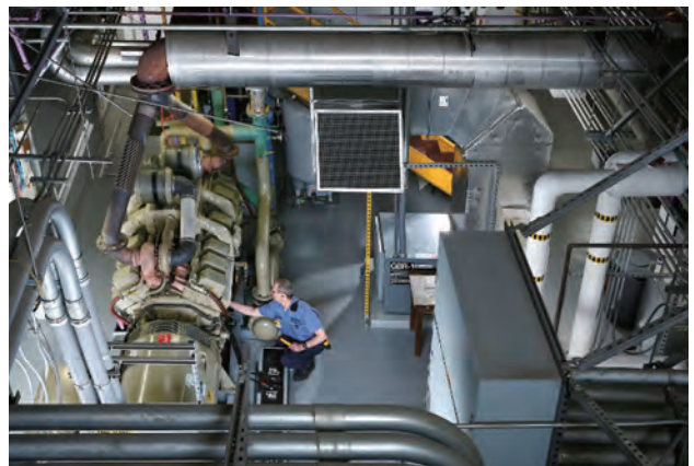
Maintenance work on power generation facilities installed in an office building basement
