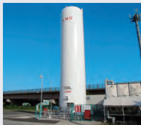
LNG satellite tank introduced at the Hokkaido plant
