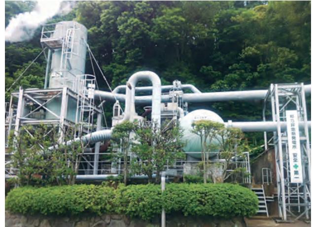
Suginoi geothermal power generation facility
