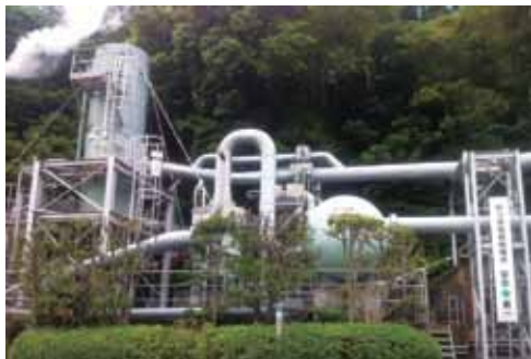
The Suginoi Hotel's geothermal power generation facility, one of largest private-use facilities in Japan
