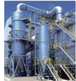
Part of Funabashi Eco Services processing facility
