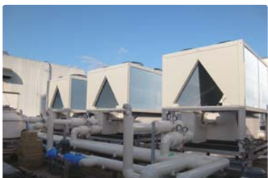
Air-conditioning equipment installed at the Nishi Kobe Factory
