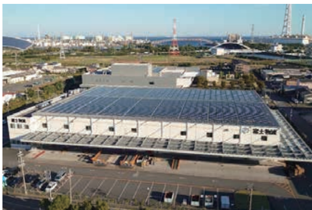
Solar power system power purchase agreement (PPA) model Fuji Logistics Co., Ltd. Mie Logistics Center
