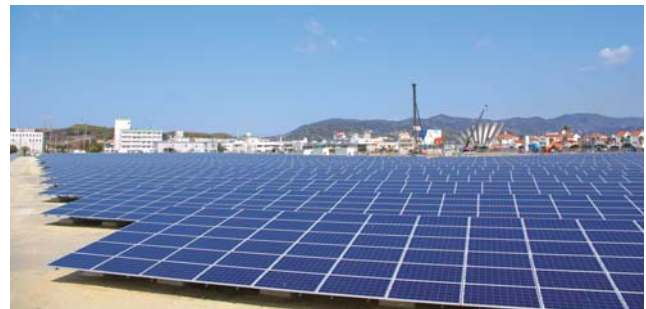
ORIX Awaji Mega-Solar Power Plant (Awaji, Hyogo Prefecture)
