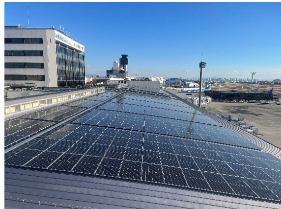
Solar power generation system at Osaka International Airport (Roof of the terminal building)
