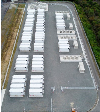
Kinokawa Energy Storage Plant
