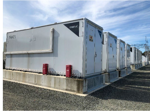
Storage battery containers
