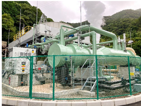
Suginoi Geothermal Power Plant
