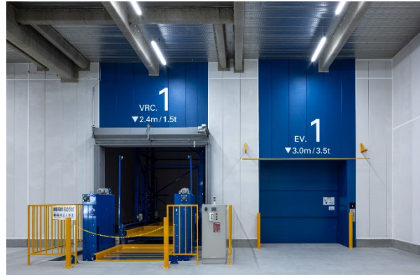
Freight elevator and vertical conveyor
