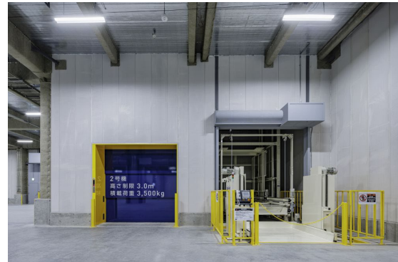
A cargo elevator and a vertical conveyor
