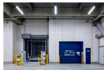
Cargo elevator, vertical conveyor
