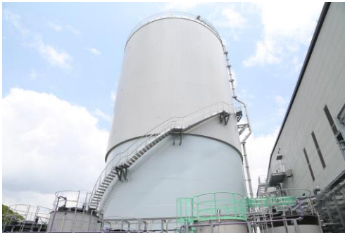
■ Methane fermentation tank
