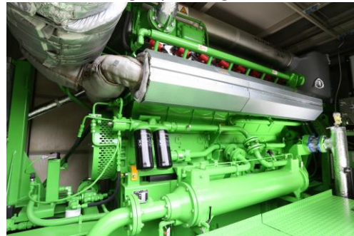
■ Biogas power generator
