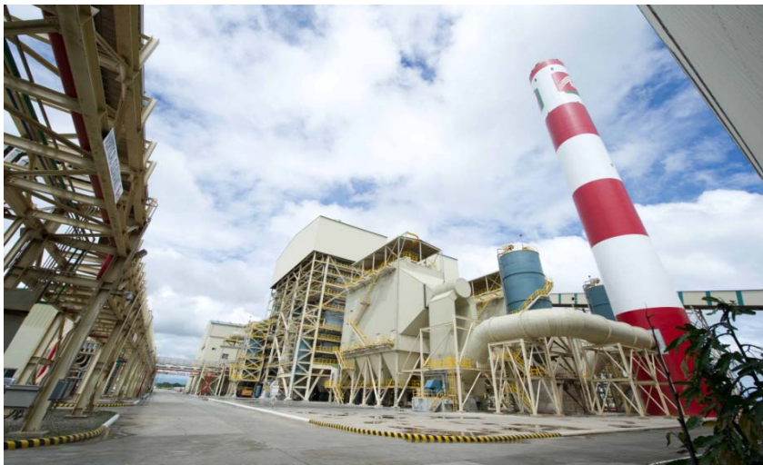
Power Plant (Panay Island)
