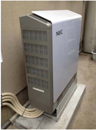
*An example of Installation to an actual detached house
