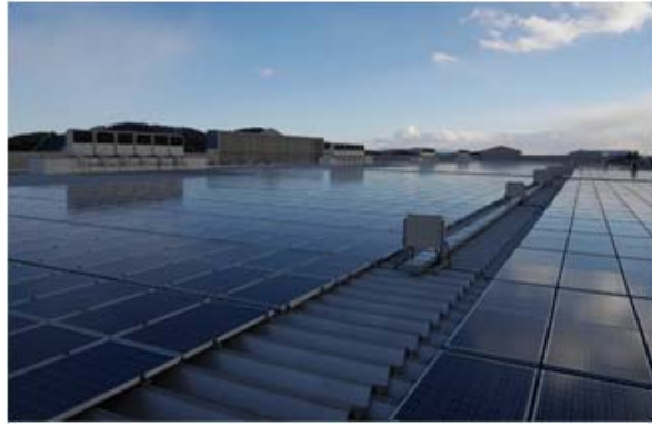
Solar power generation system installed on the roof of a retail outlet
