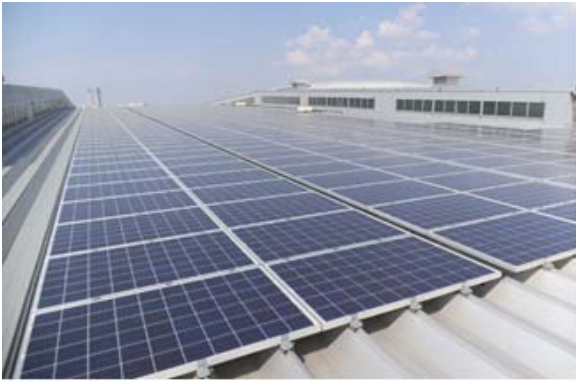
Solar power generation system installed on the roof of a warehouse
